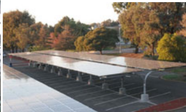
FIGURE 5 PV Panels on Shade Structure
