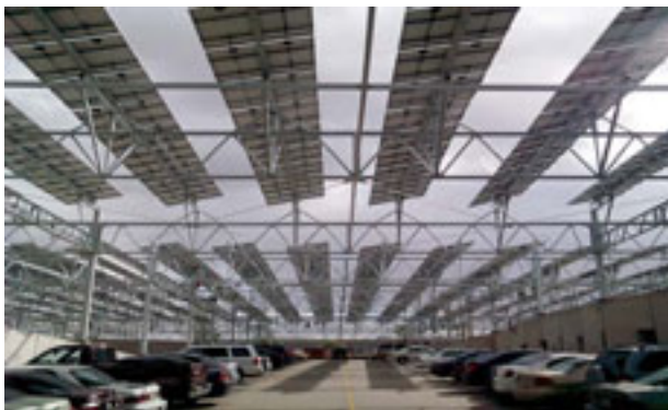
FIGURE 4 PV Panels on Structure
